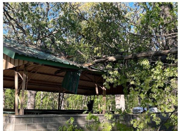
Tree damage to shelter 2 at Tyler Creek FP.
