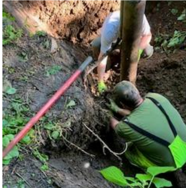
Master Tradesmen Palmisano & Guhl performing emergency well repairs at Brewster Creek FP.
