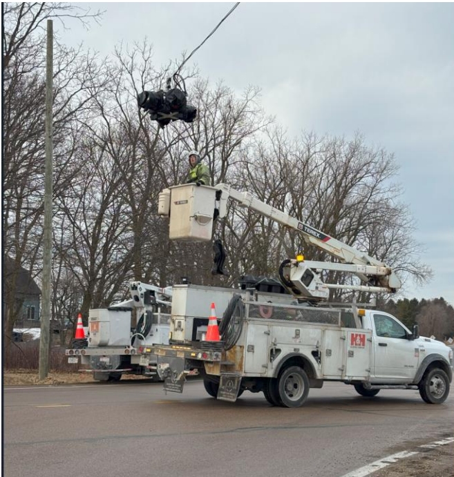
4-way overhead flashing beacon
