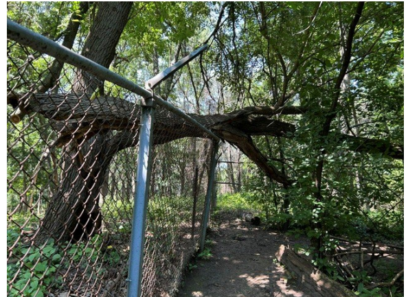
Storm damage threatens the security fencing at Schweitzer Dog Park.
